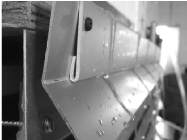
FIGURE 8: INDIVIDUAL WATER STREAMS ON THE METAL DRIP EDGE
