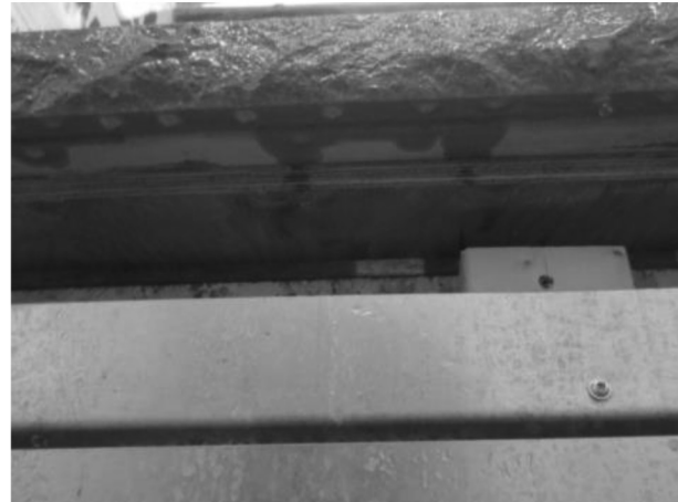
FIGURE 9: ENTIRE FRONT SURFACE OF STONE SILL IS WETTED; MANY DRIP LOCATIONS INDICATE IMPROVED HORIZONTAL DISTRIBUTION
